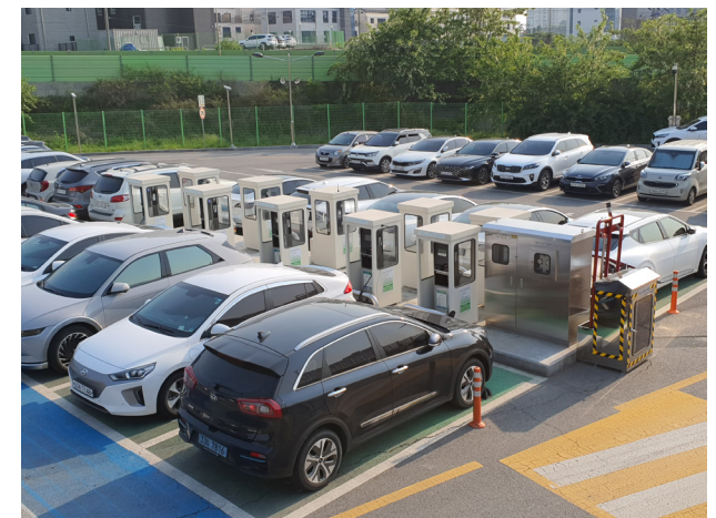
EV charging area at our Giheung worksite
