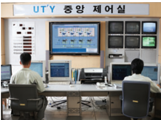
[Chiller Control System]
